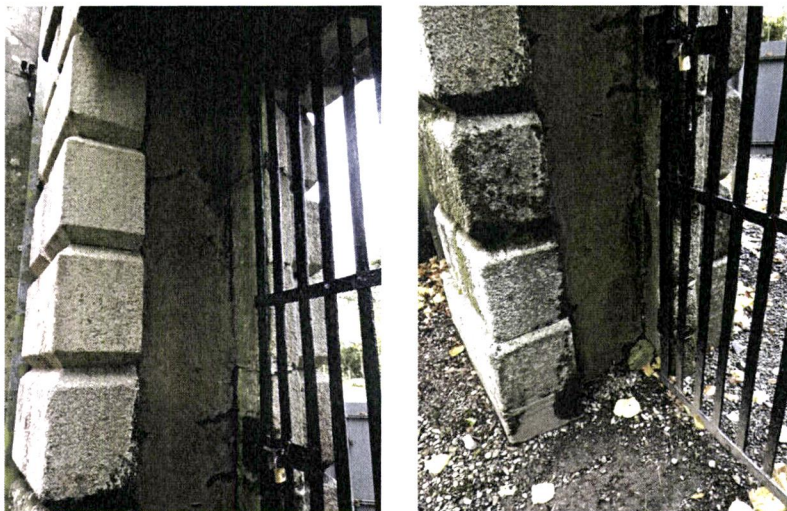
Close-up North pedestrian gateway Example of saturated and failing plaster to gate reveal.
