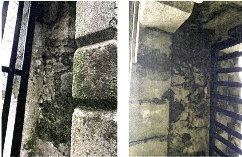
Close-up South pedestrian gateway Example of saturated and failing plaster to gate reveal.
